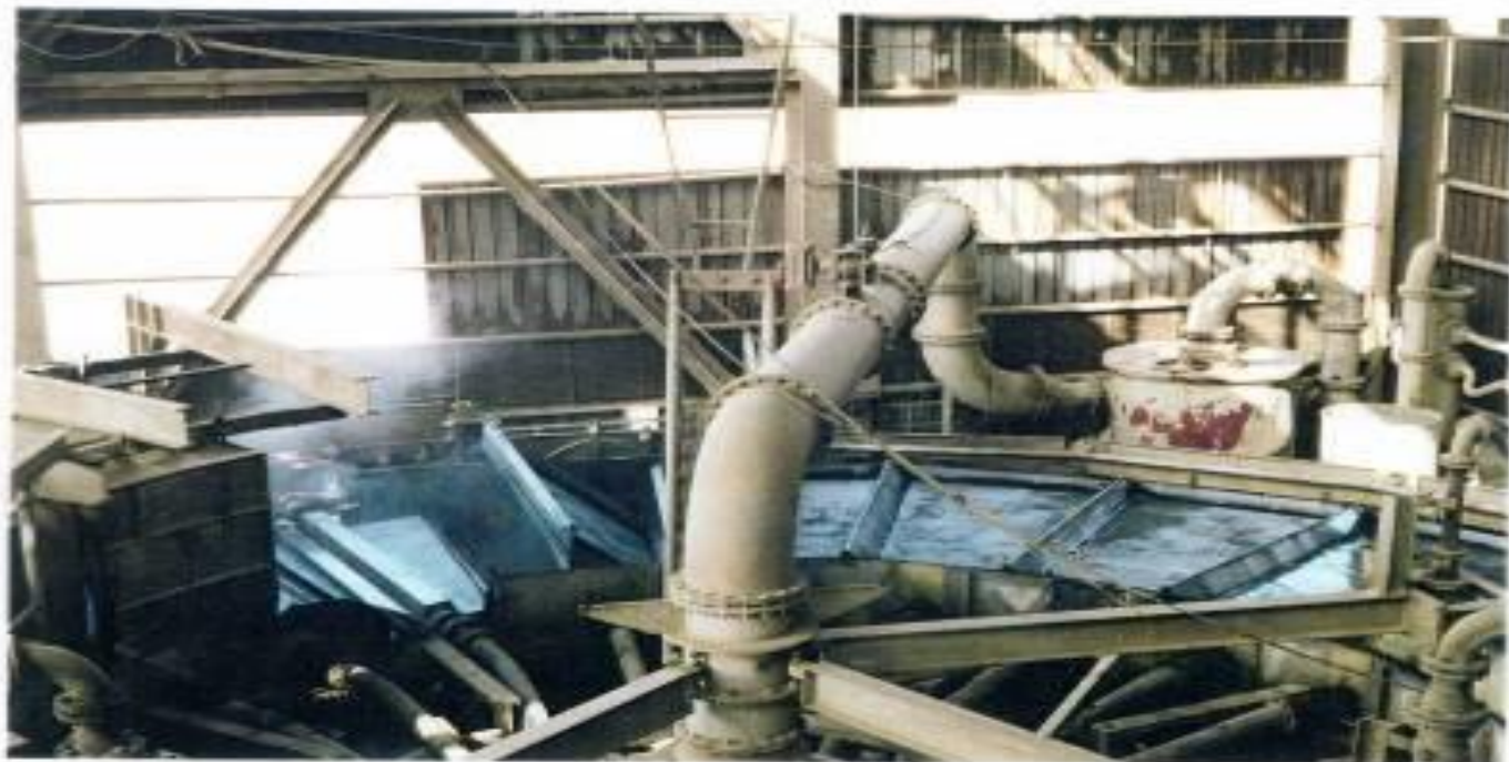
Last Stage of Gypsum Filtration
