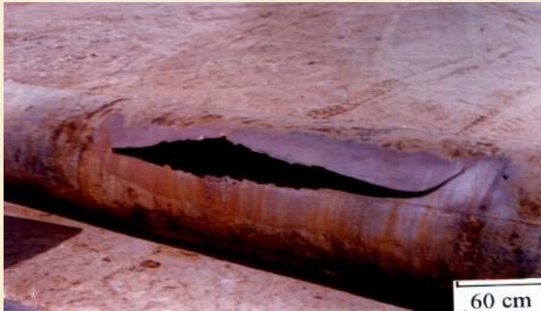
Line SUMED Pipe
