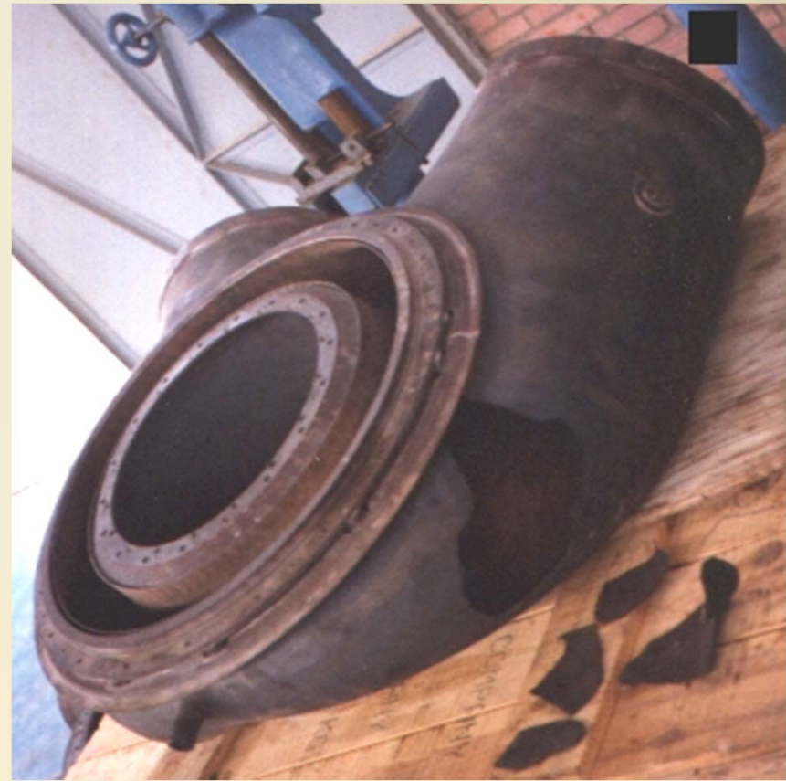
Gas Duct at GUPCO Power Station
