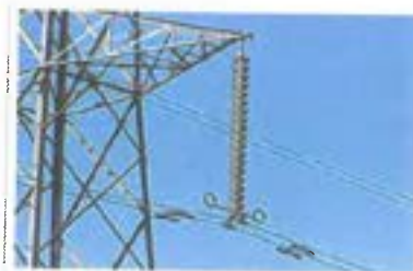
Cap and pin insulator string (the vertical string of discs) on a 275 kV suspension pylon.
